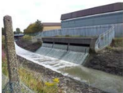
Unsatisfactory Intermittent Discharges (UIDs)
