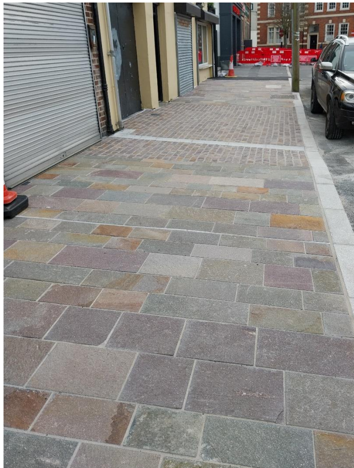
A section of completed footway at the north end of The Square
