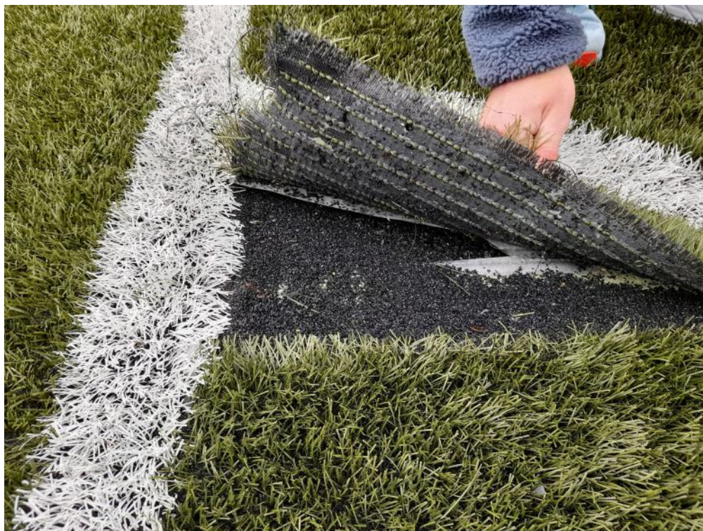
16 – Open Joint/ Seam
