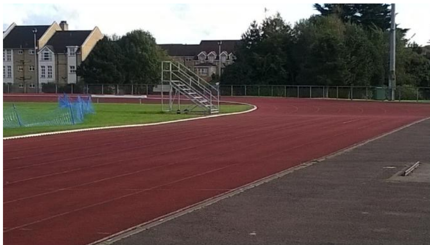
Photo 13 – Depression at finish line
