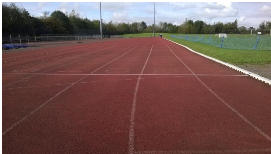
Photo 12 – Depression at finish line
