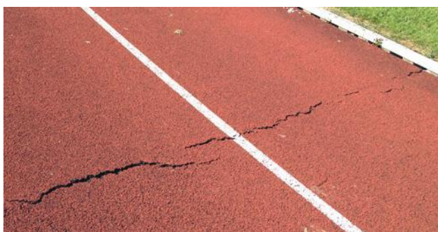
Clearly apparent cracks
