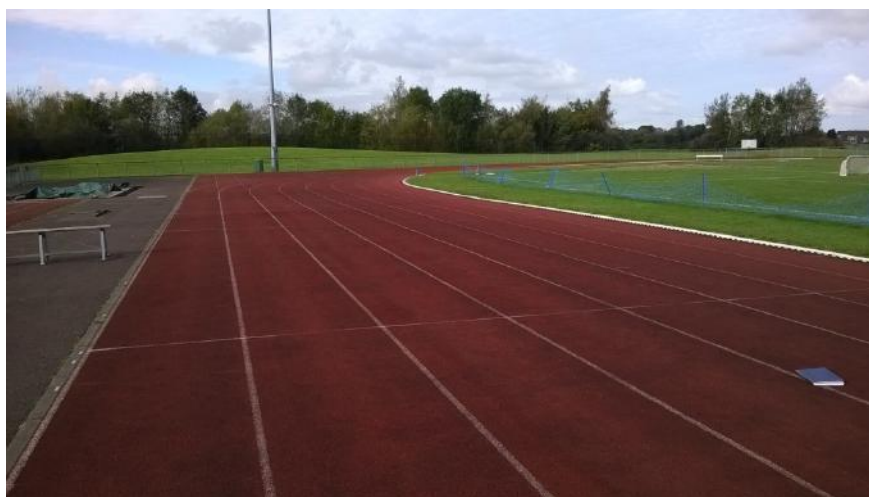
Photo 14 – Depression at start of home straight
