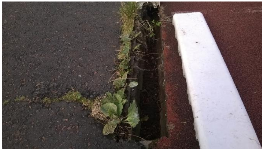
Photo 5 – typical weed growth at drainage channel
