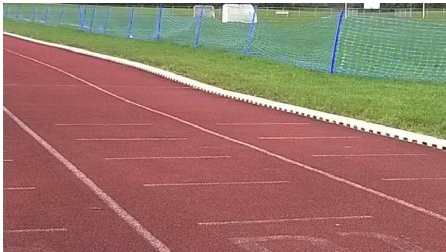
Photo11 – Depression at finish line
