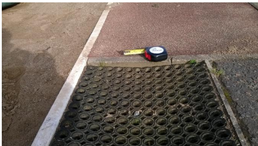
Photo19 – Depressions in safety matting
