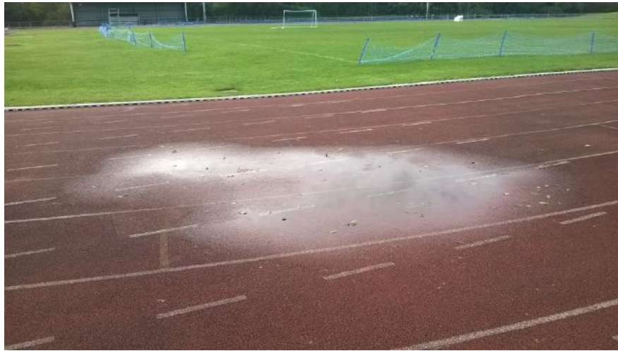
Photo 8 – Depression and ponding at start of back straight.
