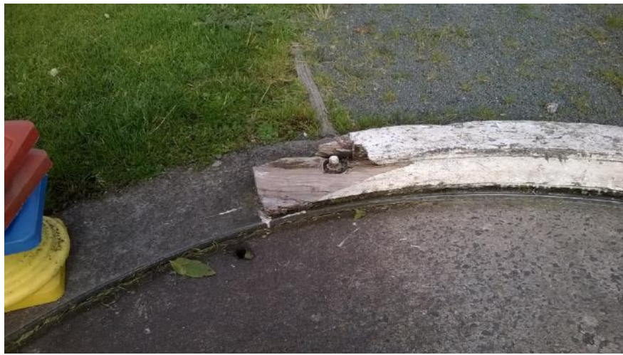
Photo 37 – Damaged throwing board.
