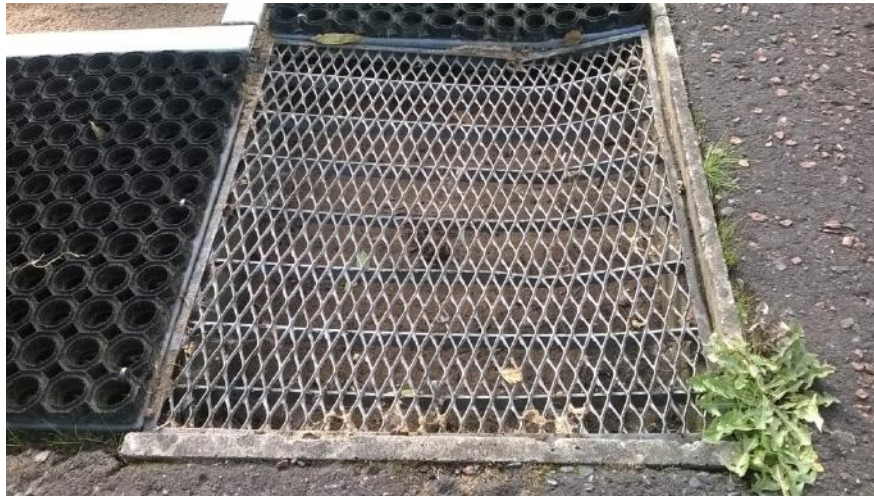
Photo 21 - Depressions in safety matting
