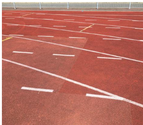
Figure 4 Widespread patching at an area of noted settlement at start of back straight
