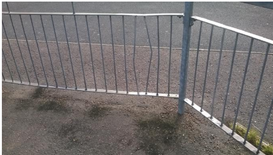
Photo 2 – Localised damage to fence at south west end of track
