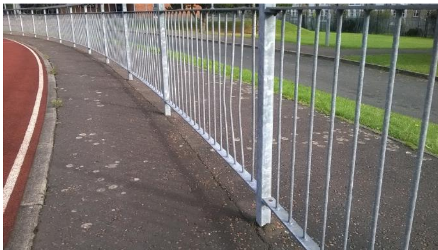
Photo 3 - Localised damage to fence at southern end of track
