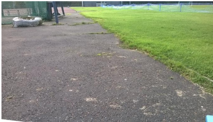
Photo 23 – Settlement in bitmac
