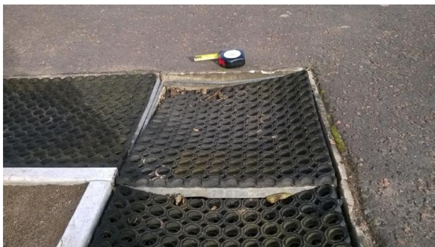
Photo 20 - Depressions in safety matting
