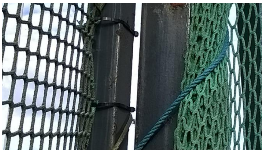
Photo 25 – Corrosion of steel members at throwing cage.
