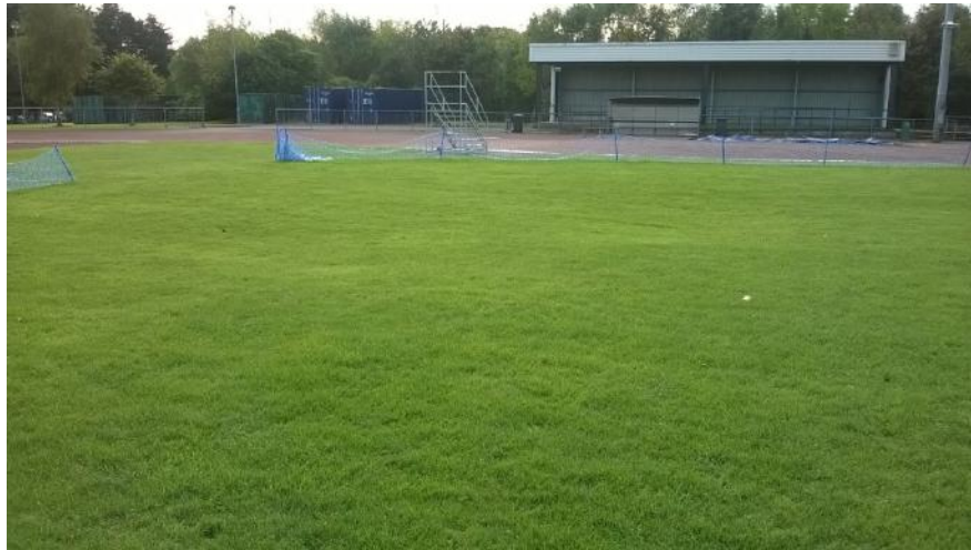
Photo 42 - Settlement in track infield
