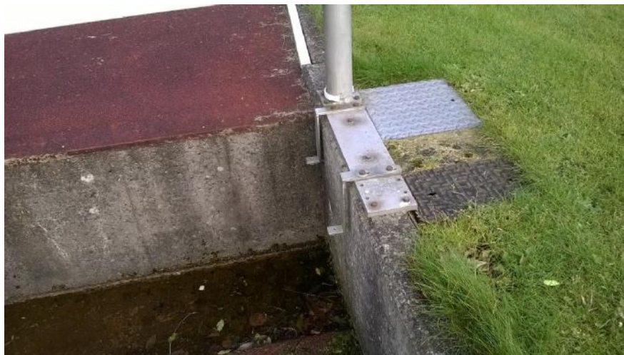
Photo 35 – Steeplechase water jump protruding brackets
