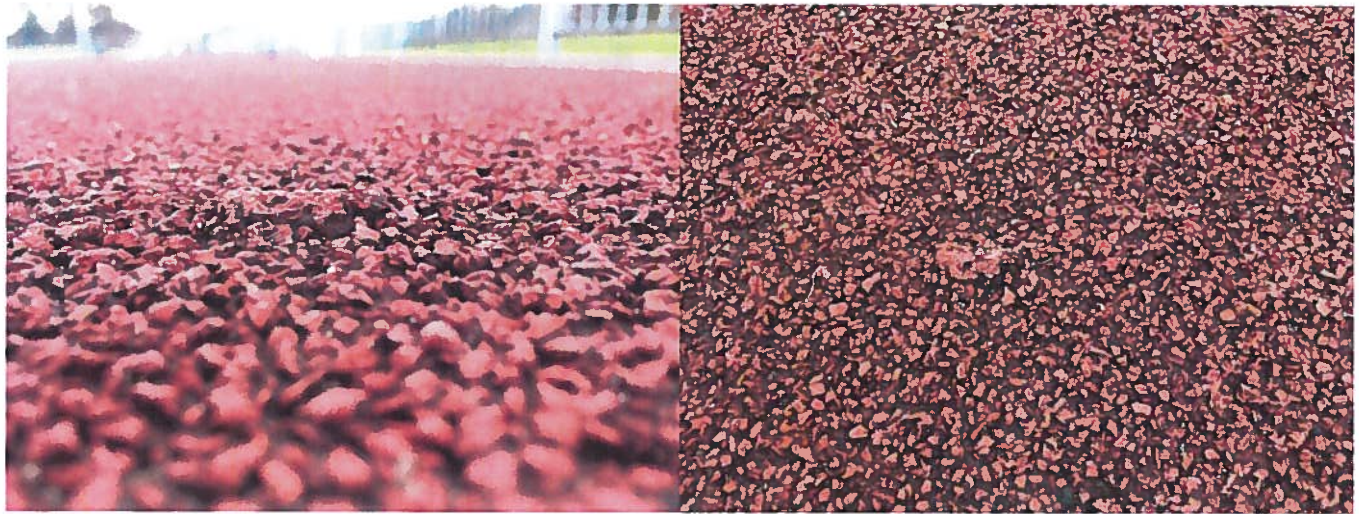
Areas of fissures and bubbling causing point undulations across the track
