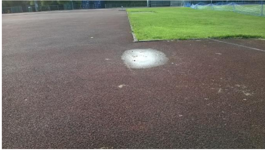
Photo 34 - Depression at Javelin runway.
