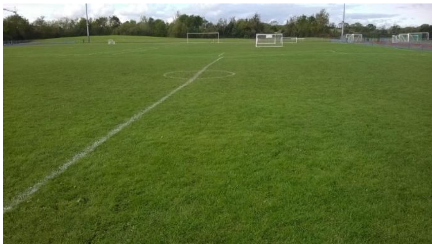
Photo 44 – Settlement in track infield
