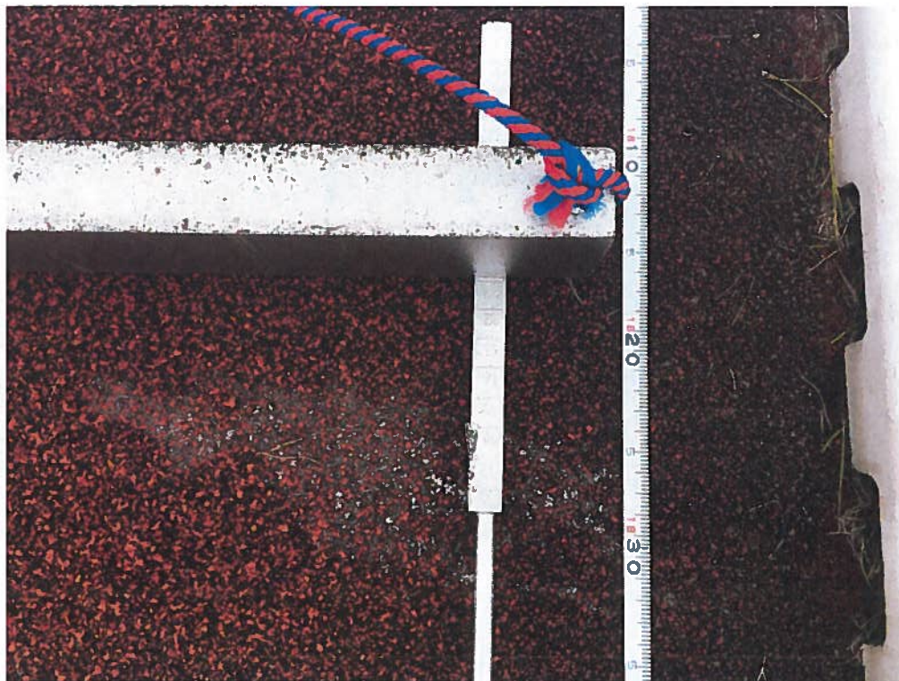
Continuous undulation where track drops into inside lane kerb
