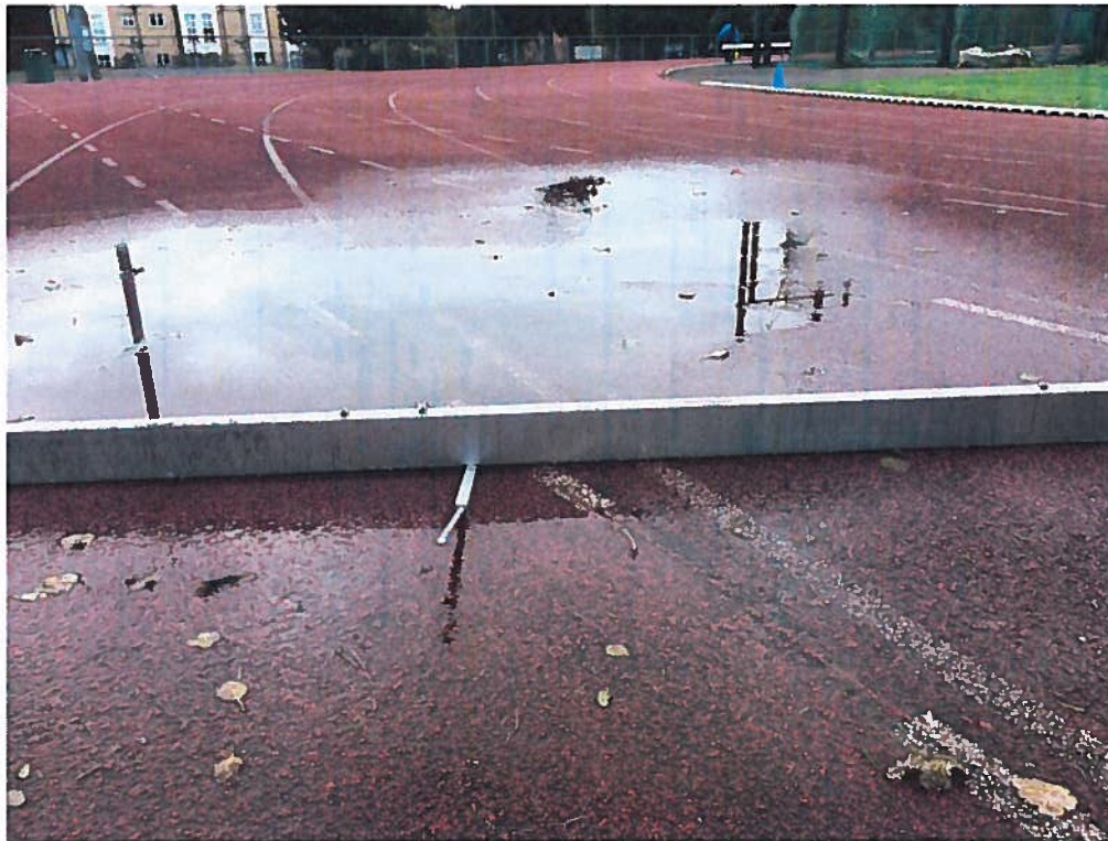
Significant undulation on S-E track bend creating an area of standing water
