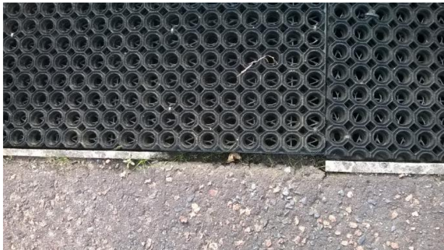
Photo 22 – Long Jump pit north end missing kerb.
