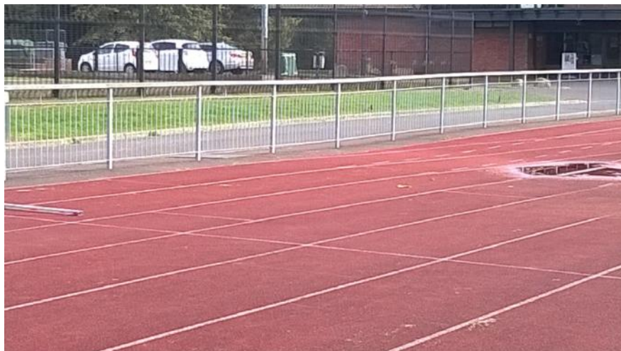
Photo 9 - Depression and ponding at start of back straight.
