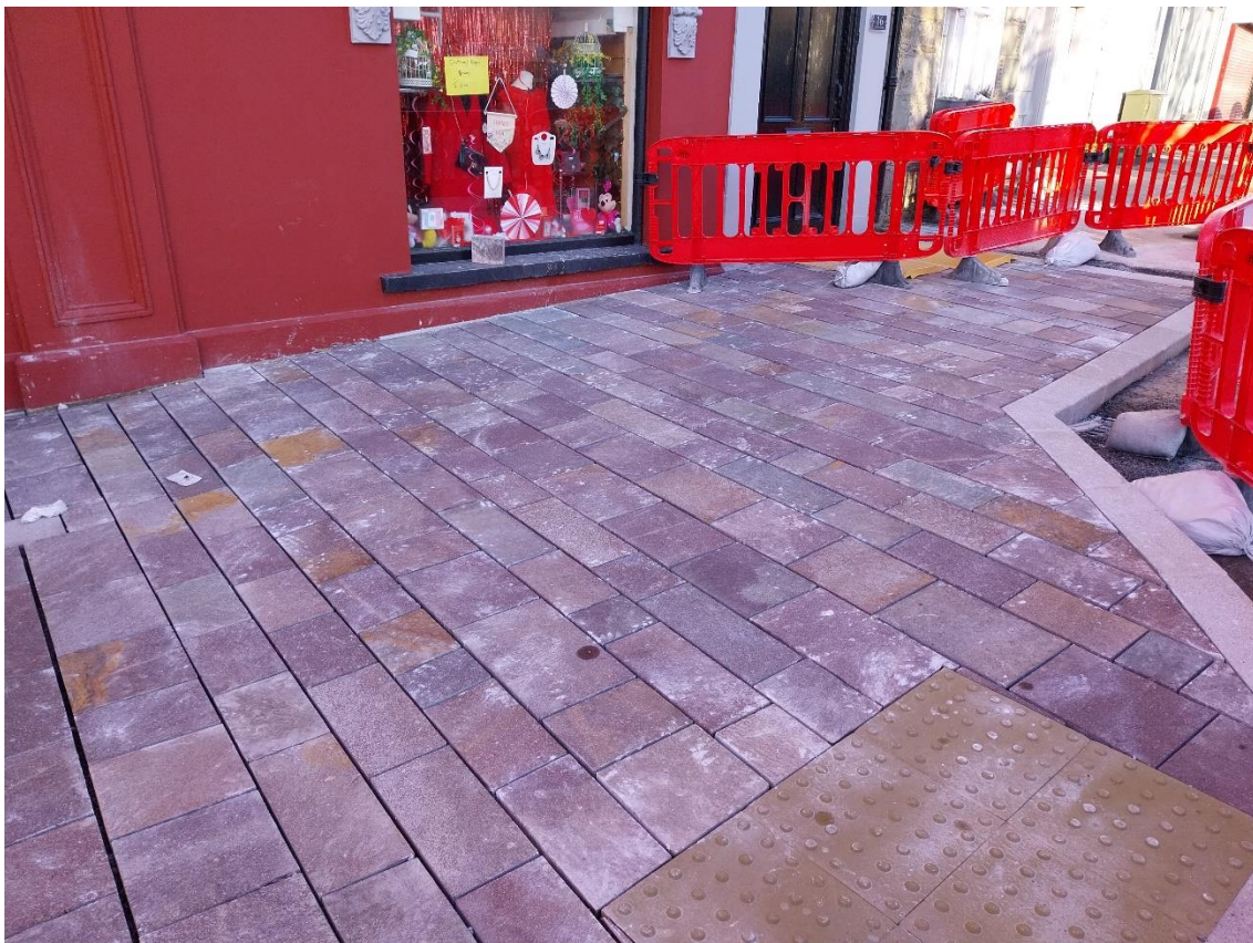
New paving works on the west side of The Square outside No.16
