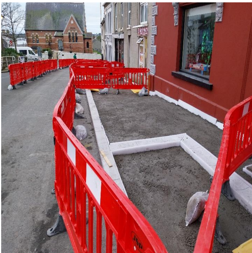
New granite kerbing installed to the side of Market Square, and concrete base laid in advance of the paving works which are due to start in February
