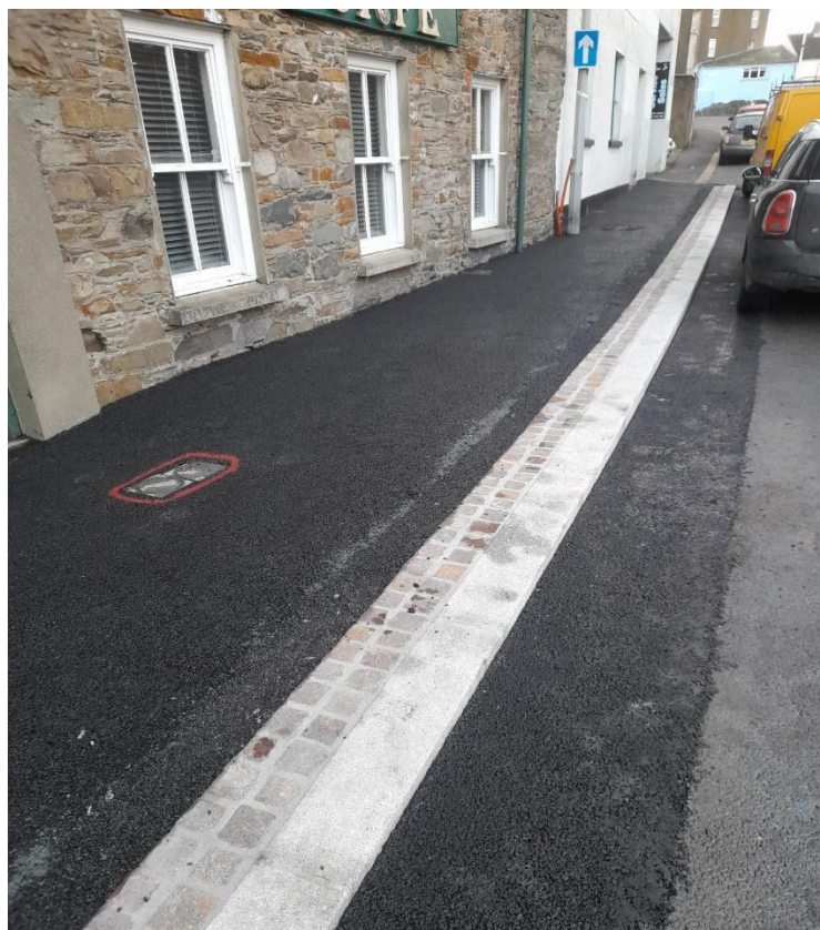
Works progressing on Castle Street with the base material and porphyry band laid
