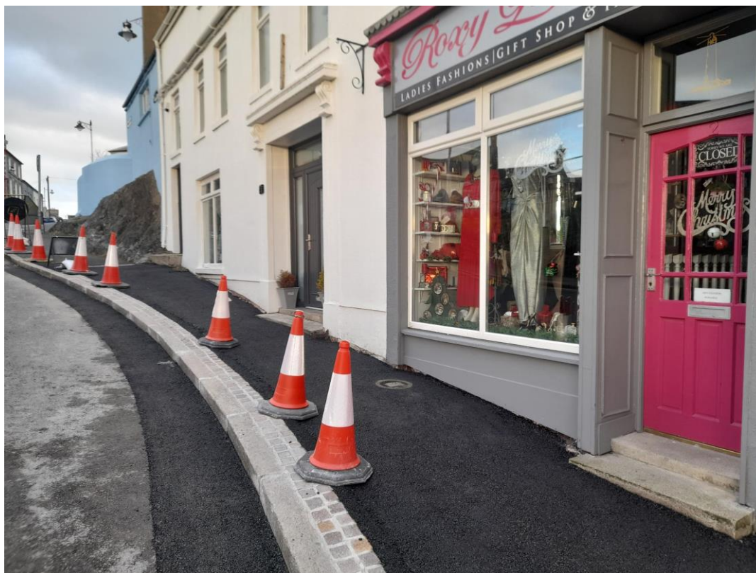
Works progressing on Ferry Street with the base material and porphyry band laid
