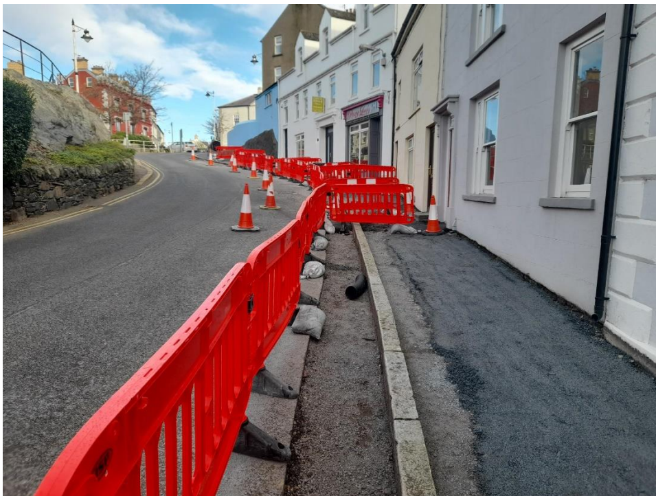
The re-laid pavement at Ferry Street awaiting the Italian Porphyry stone band placement to be installed on the left section of the above pavement image
